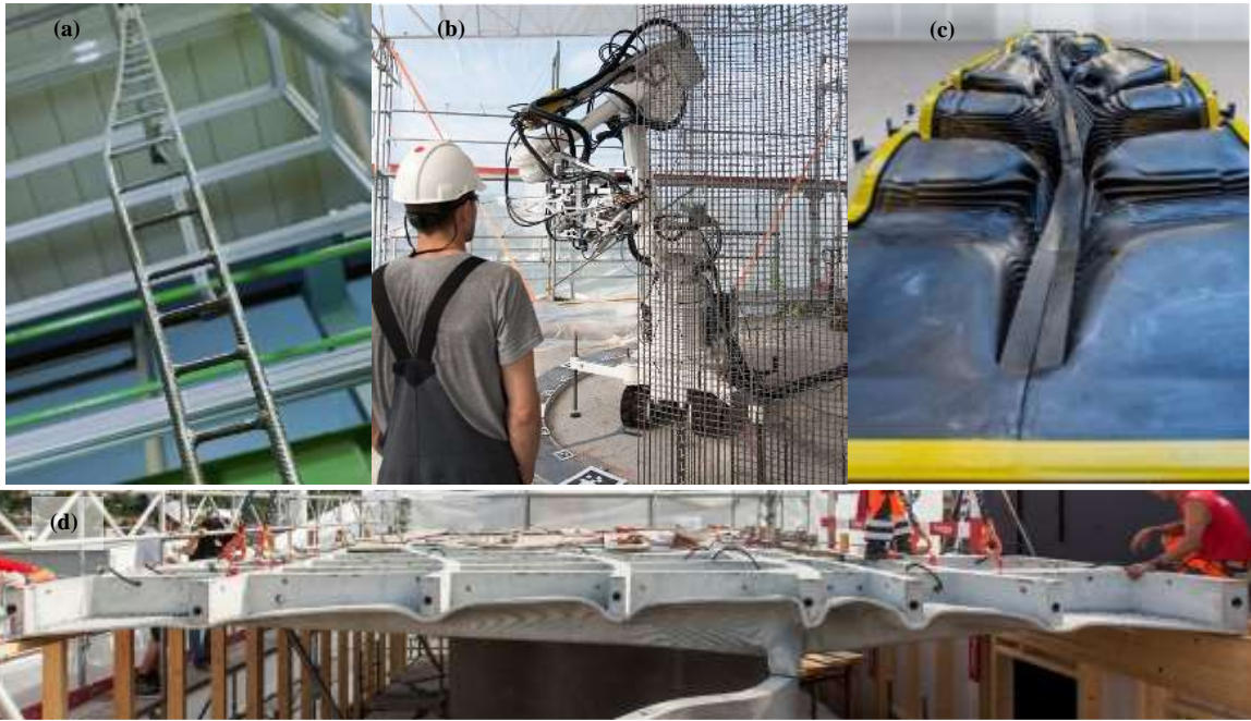
5 6 Figure 3. Details of production of concrete structures for the DFAB HOUSE: (a) reinforcement of the mullions installed 7 prior to concrete production [90]; (b) on-site robotic fabrication of double curved reinforcing mesh [42]; (c) 3D-printed 8 formwork for a 7.1-m segment of the Smart Slab [91]; (d) installation of the prefabricated Smart Slab [91].
