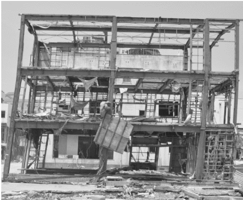
Figure 1 - Global deformation of MR- steel frame after an earthquake [Gioncu and Mazzolani, 2014]
