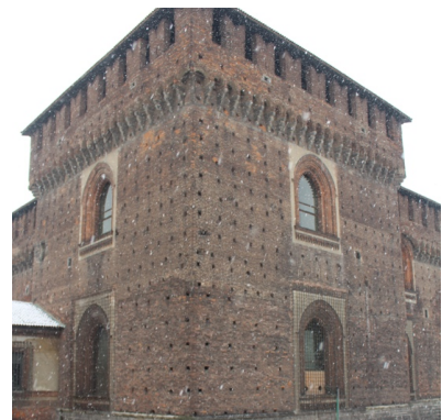
Figure 1: the Falconiera tower and its affected windows.
