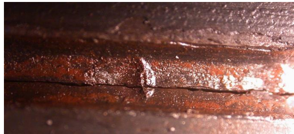
Figure 6. Enlargement of the circumferential view of the crack
