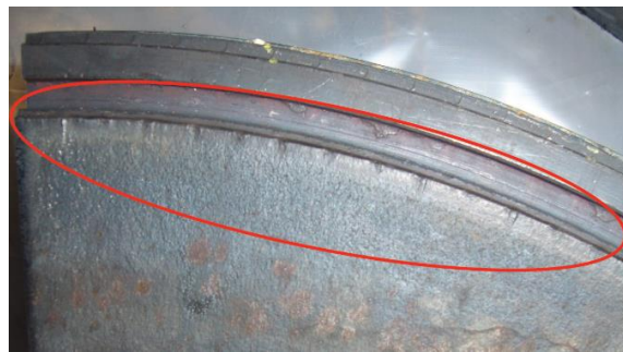
Figure 11. Multiple initiation points of the crack
