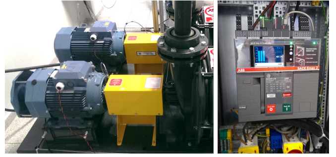
Fig. 2. Pictures of the experimental setup. Left: induction motors employed for the tests. Right: Emax2 ® breaker installed in the electric cabinet of the testing laboratory.
