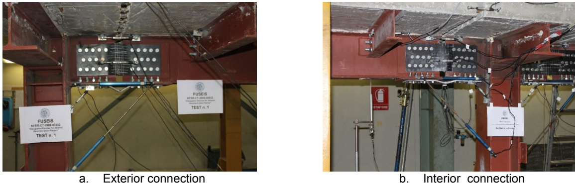
347 Figure 16 Inelastic deformation of the structural fuses
