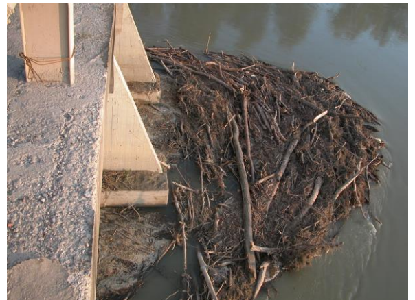
Figure 2. Clogging phenomenon on a bridge over the Po River, Guastalla, Italy (Malerba, et al. 2013).
