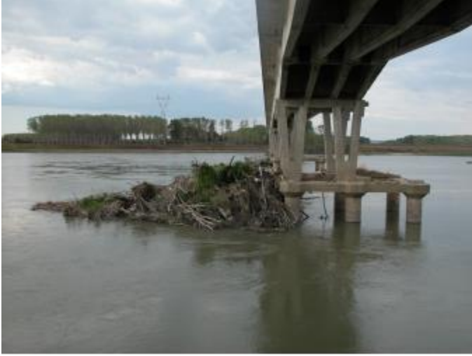
Figure 1. Clogging phenomenon on a bridge over the Po River, Pieve Porto Morone, Italy (Malerba, et al. 2013).
