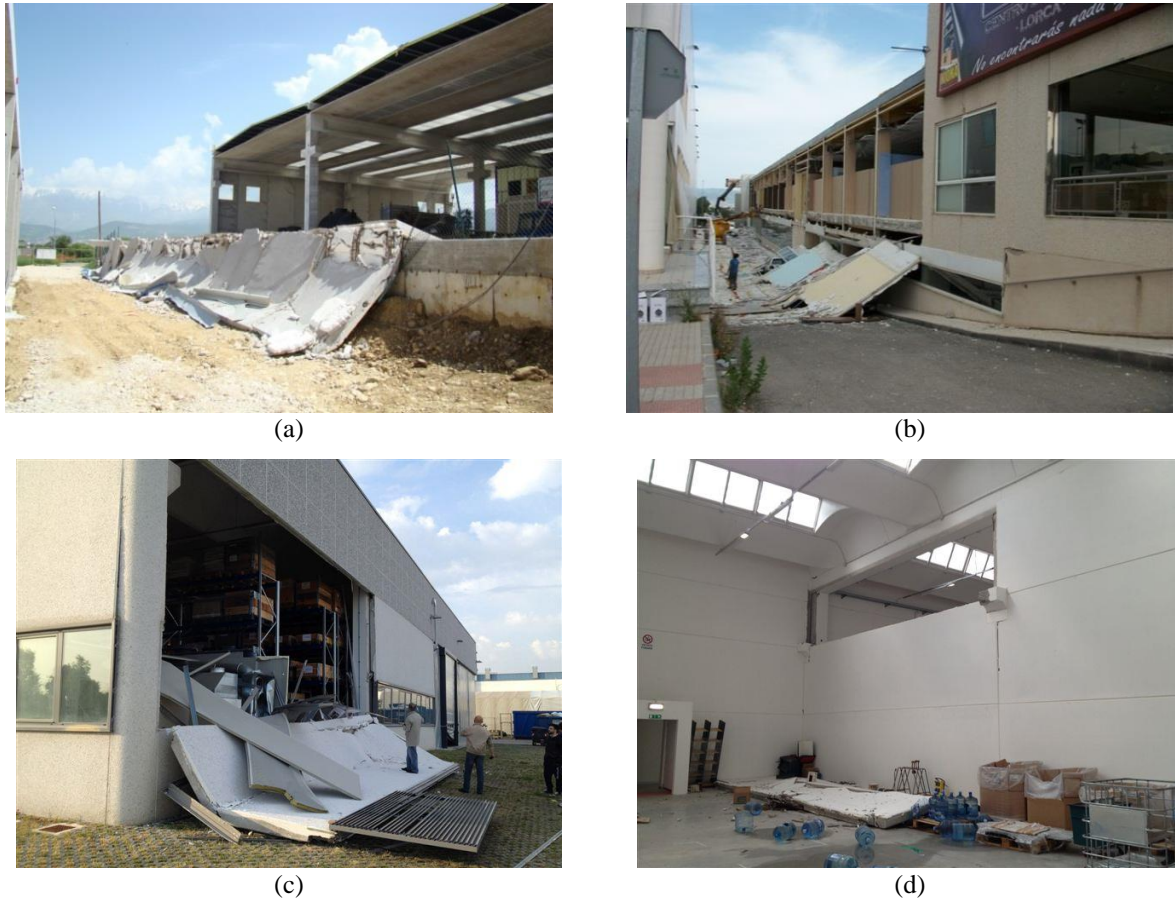
Figure 2. Failures of cladding panels through earthquakes: (a) L'Aquila 2009, (b) Lorca 2011, (c,d) Emilia 2012
