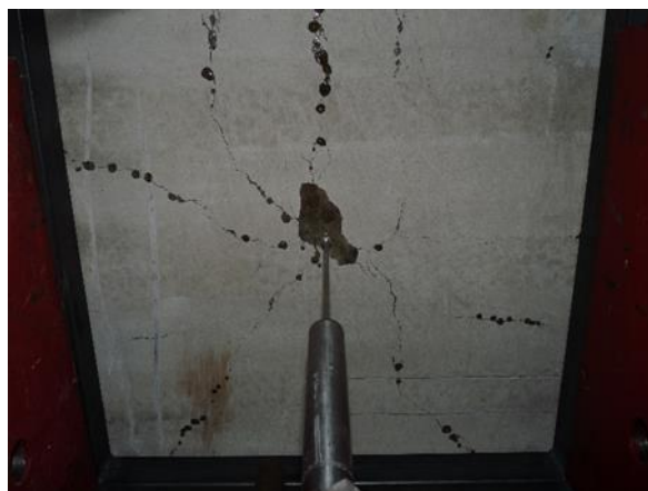
57 58 Figure 15. 2D vascular network releasing sodium silicate in a 600mm square concrete slab. 59 60 61 62 63 64 65
