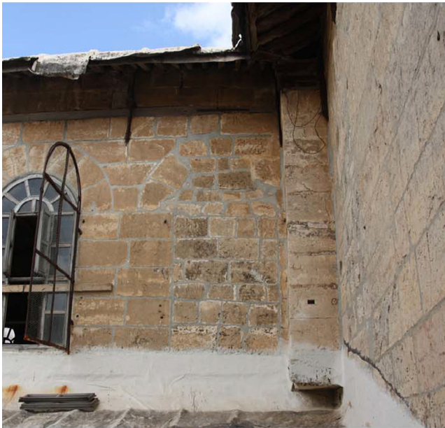
Fig. 15. Buffered window of the nave at the intersection with the transept wall.
