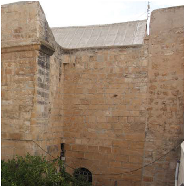
Fig. 19. Buttress added as a protection of the Western wall of the North transept.
