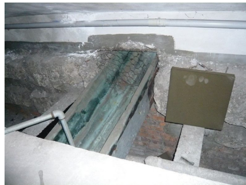
Fig. 5. Brera Palace, Milan. The connection of the water duct from the eave gutter to the downspouts. A metal grid protects the obstruction of big objects.
