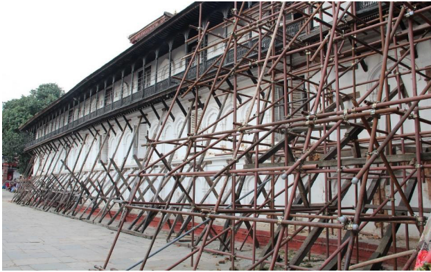
Fig. 10. Earthquake damaged heritage building in Nepal supported by poles and scaffolding.
