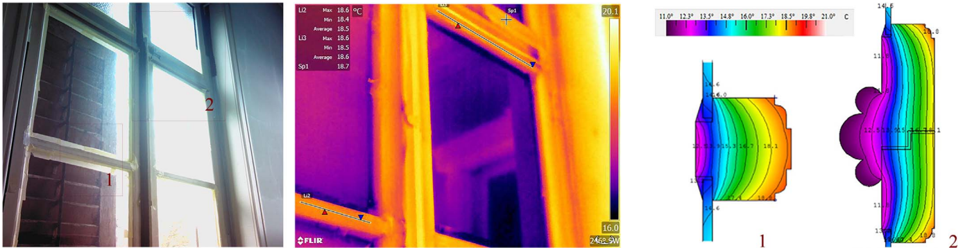
Fig. 3.3.3. (a)–(c) Central window frame connection; from the left (a) transom localization, (b) IRT imaging, (c) window model (THERM 7.4).
