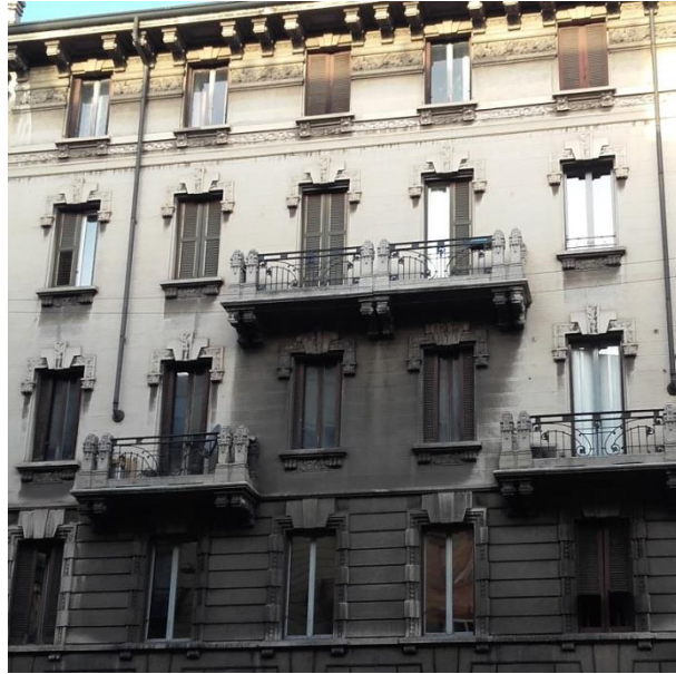
Figure 5. The façade of a building in Milan, showing the impact of morphology on soiling (please note that this façade is not covered with the materials investigated in this study. It is shown with the only purpose of demonstrating soiling patterns on complex façades).
