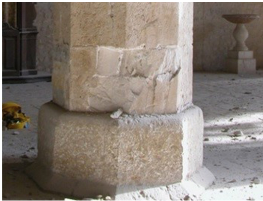
Fig. 17. Earthquake damage at the base of the column.
